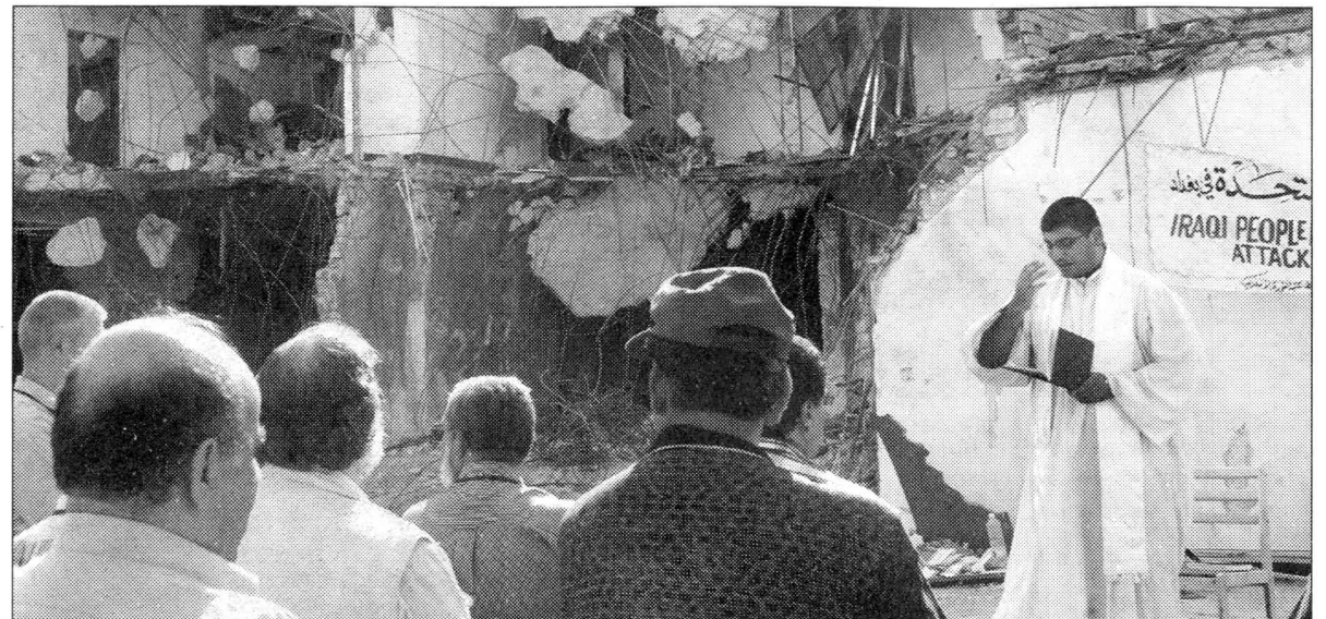
U.N. staff are led in prayer by a Christian pastor from the Chaldean church in front of the devastated former U.N. headquarters in Baghdad, the scene of a massive car bomb, during a memorial service on August 30. The bomb on August 19 killed 22 people, including the U.N. envoy Sergio Vieira de Mello. REUTERS
