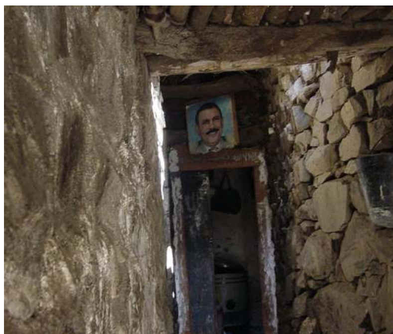
Beside the 21 houses that were destroyed, other houses are subject to collapse and have cracks in their walls.
