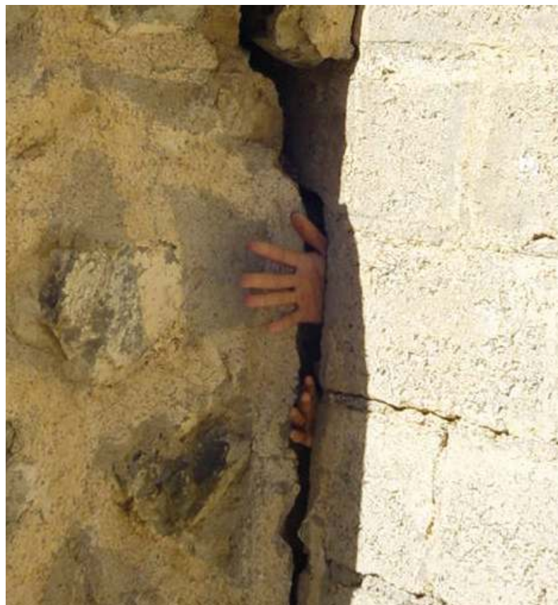
Houses in the village are not suitable to be lived in after the landslide and might collapse at any moment.
